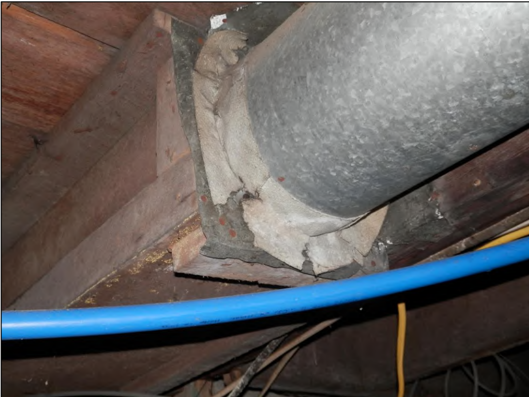
PHOTO 14: Asbestos containing seam tape insulation in basement
