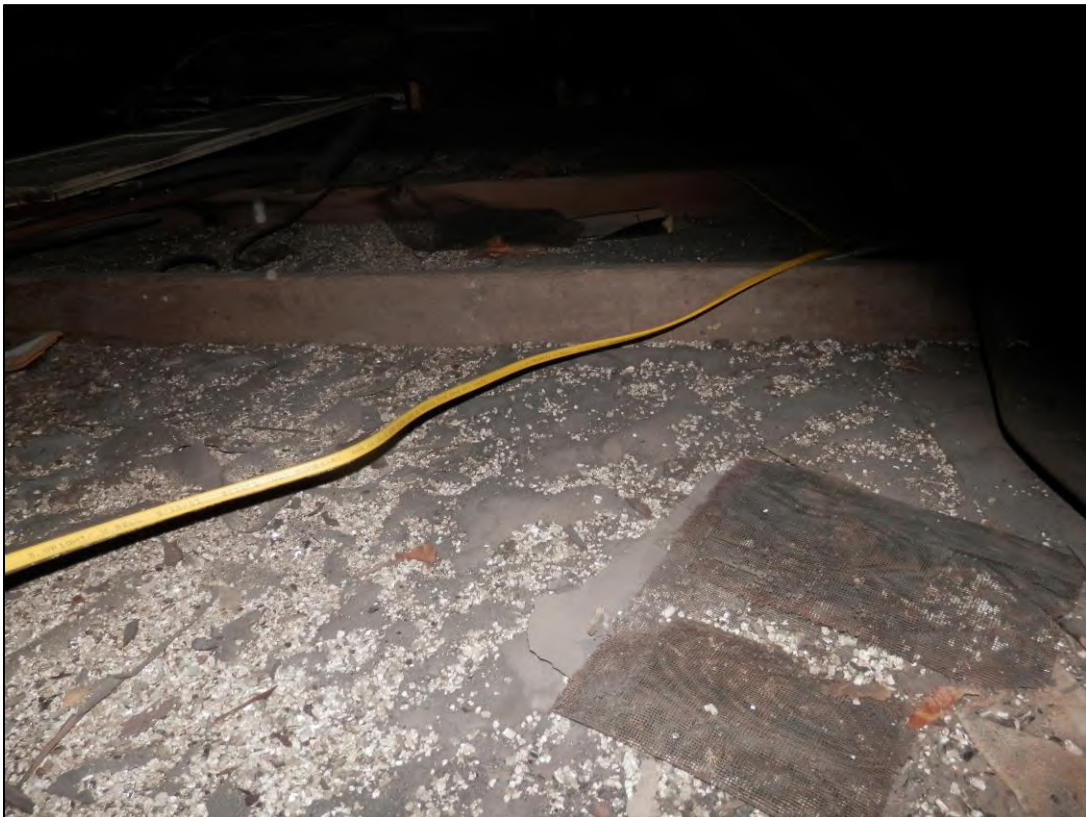
PHOTO 16: Residual loose-fill vermiculite in attic
