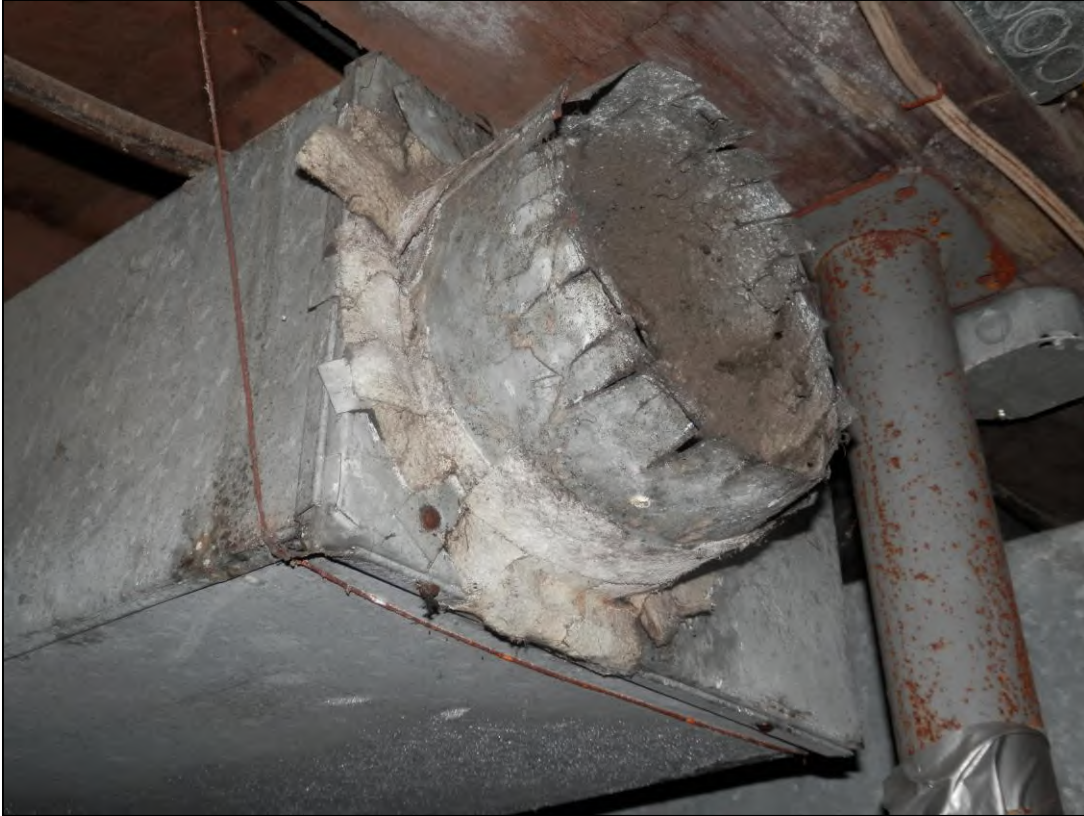
PHOTO 13: Asbestos containing seam tape insulation in basement
